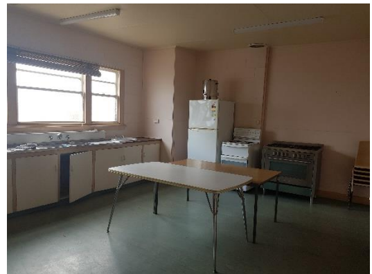
Image 7: Downstairs Kitchen Facilities 1 of 2
