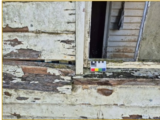
10. Rotting weatherboards and windowsill.
