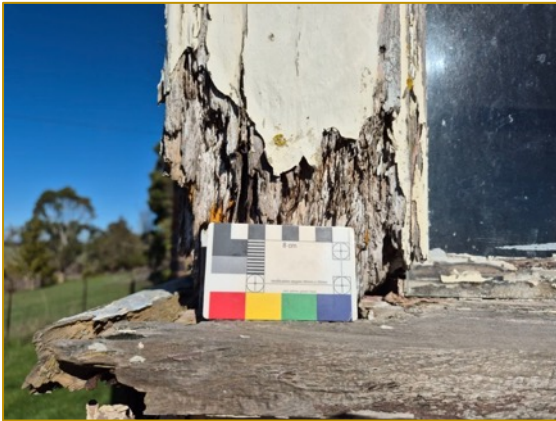
9. Weather damaged window,
