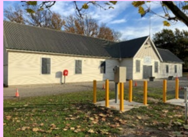
Contractors were engaged to remove weathered, rotten weather boards and replace with new at Fall Park in Evandale.
