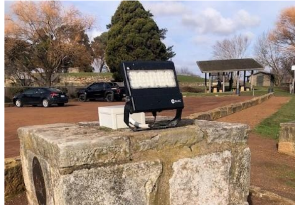
Ross Bridge flood light
