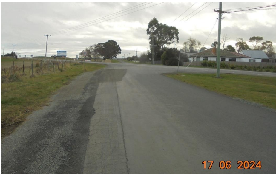
^Intersection of West Street and Midland Highway with widening required for the quarry permit
