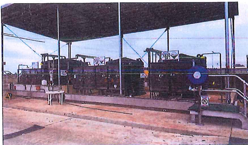
Figure 13 - Chemical storage and dosing facility at Kingaroy
