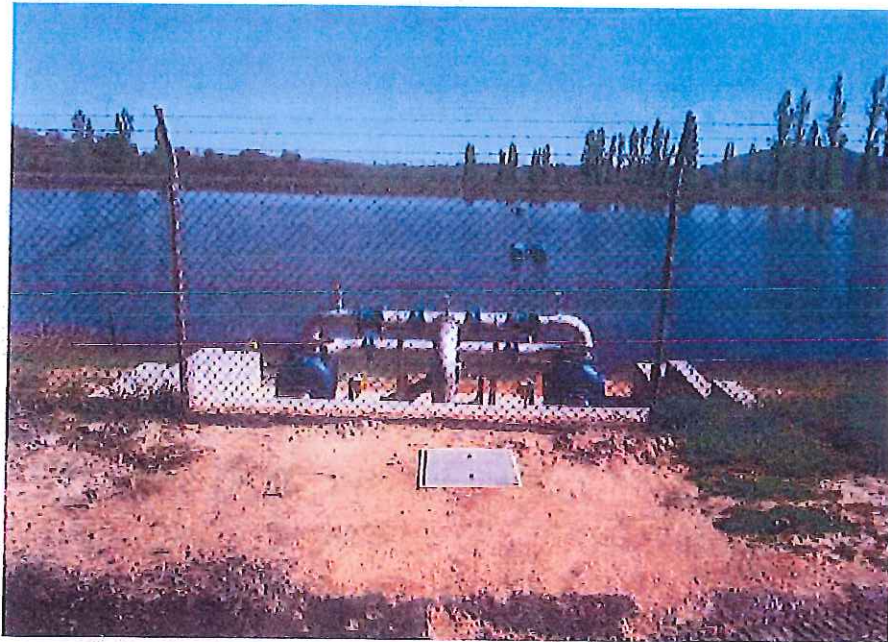
Figure 8 - Typical Lagoon return pumps
