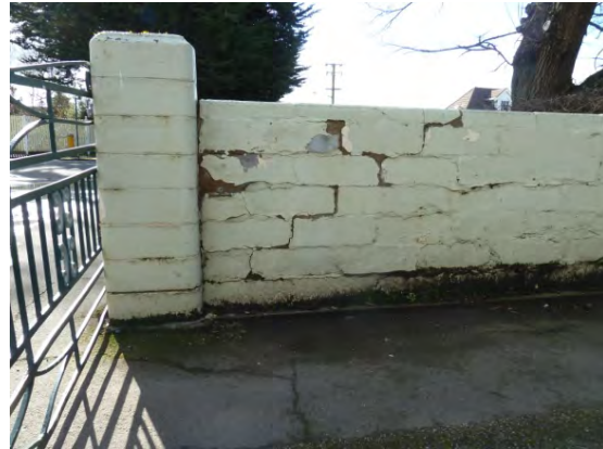
89 Fence to be replaced
