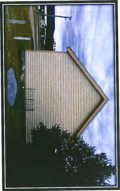
Southern End Rear Wall
